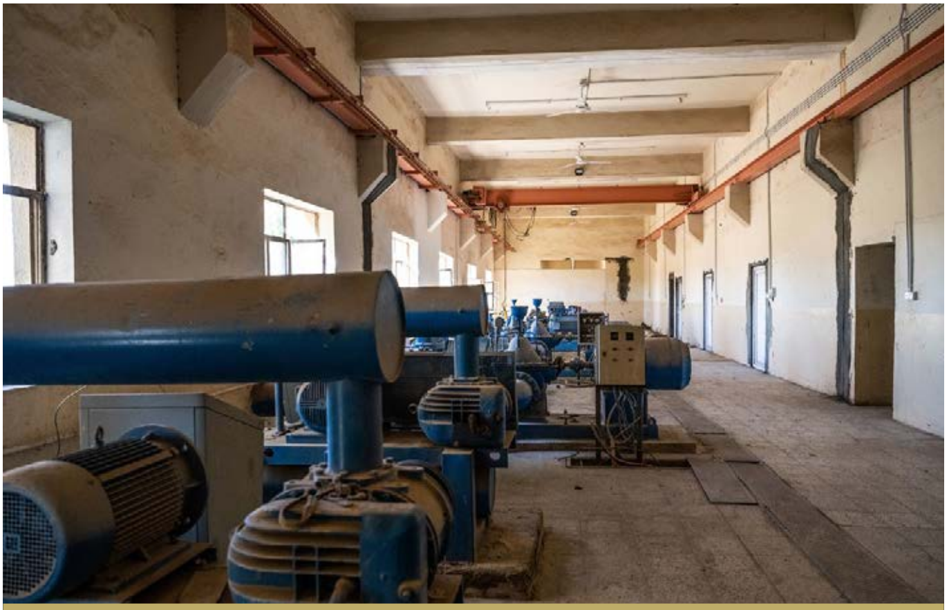
WORK ON THE HAWIJA WATER TREATMENT PLANT STARTED IN 2018 AND WAS 1% COMPLETE BY THE END OF THE YEAR.
