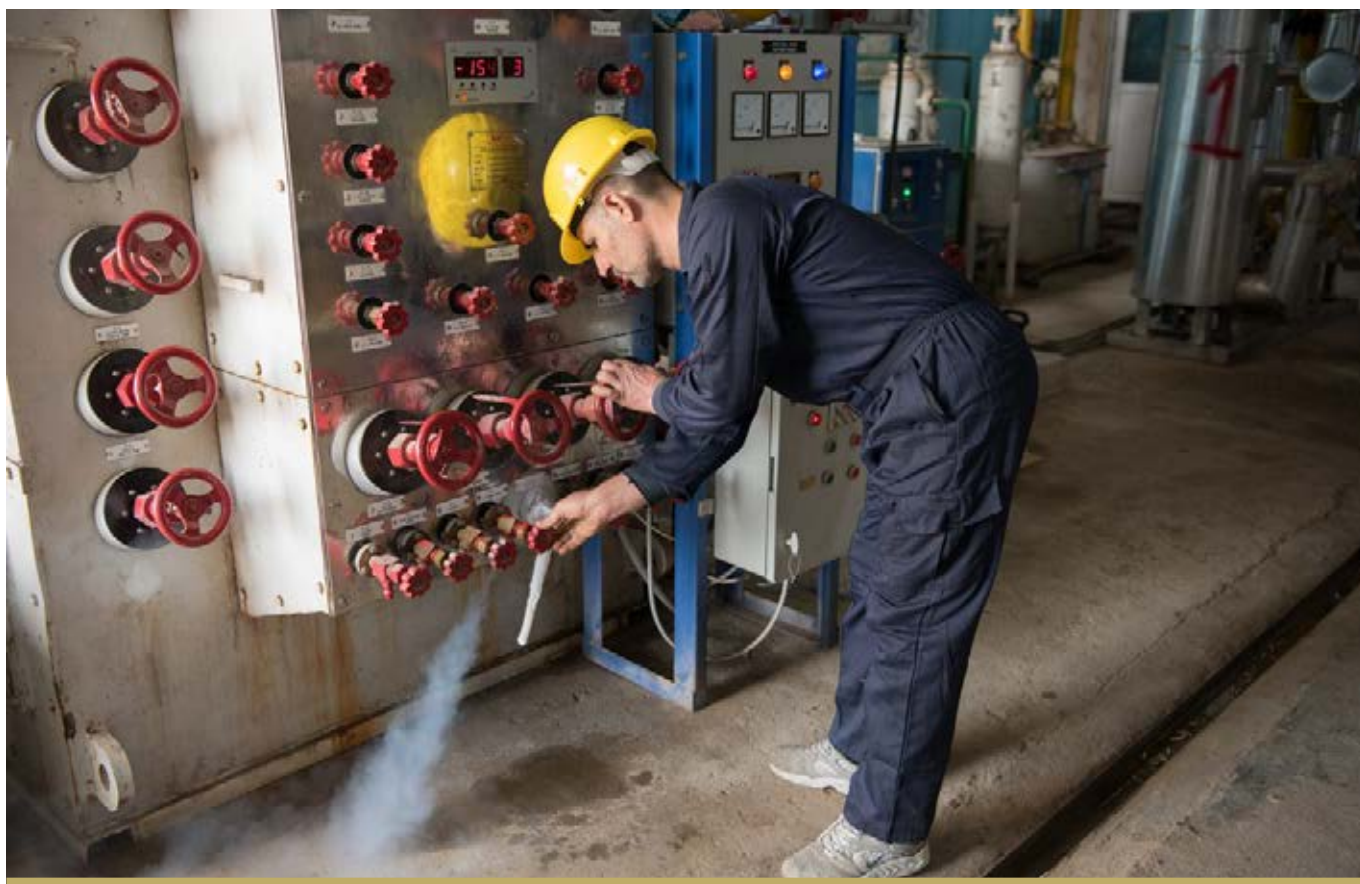
AN OPERATOR WORKS AT THE MEDICAL OXYGEN GAS PLANT AT THE TIKRIT TEACHING HOSPITAL. THE REHABILITATION OF THE GAS PLANT WAS COMPLETED IN 2018.
