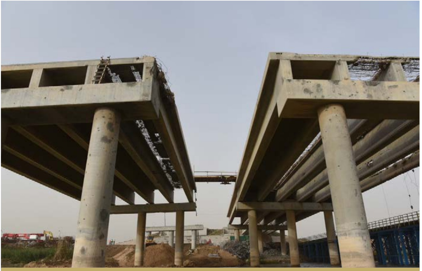
BOTH SPANS OF THE JAPANESE BRIDGE ARE BEING REHABILITATED BY THE FFS, AND THE PROJECT WAS 21% COMPLETE BY THE END OF THE YEAR.
