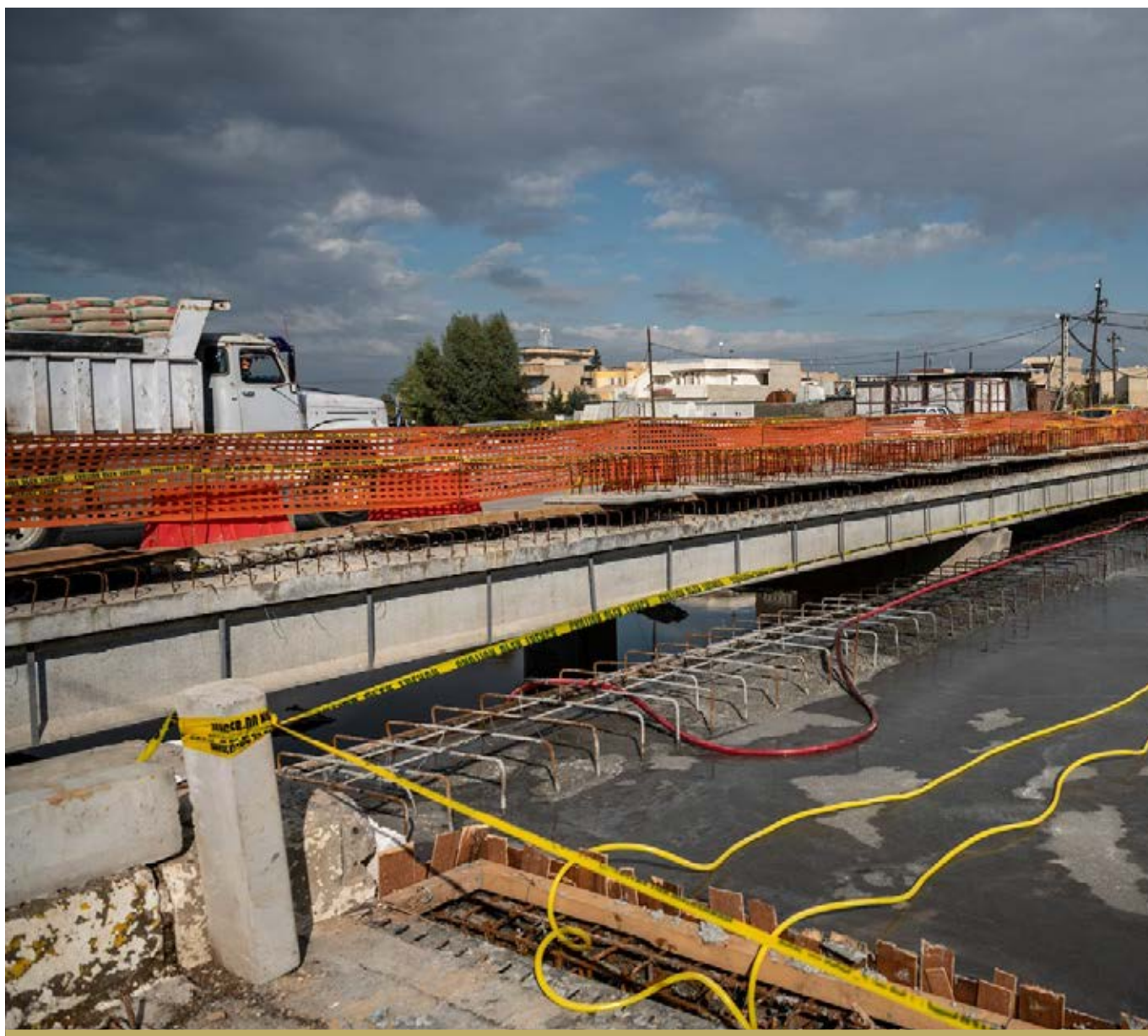
THE ASSESSMENT AND DESIGN FOR AL SUKR BRIDGE WAS UNDERTAKEN IN 2018 AND THE PROJECT WAS 85% COMPLETE BY THE END OF THE YEAR.
