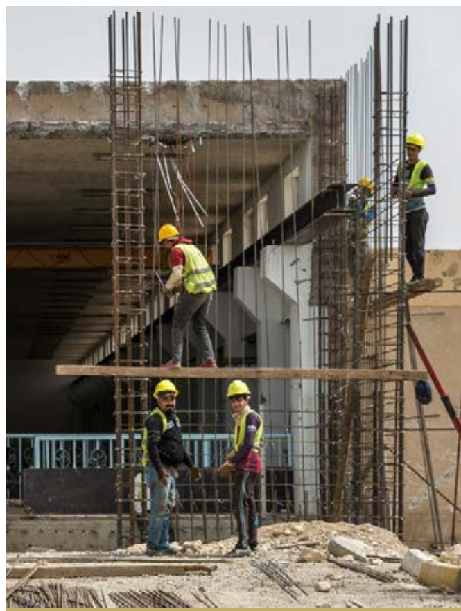
WORK IS ONGOING AT THE NEW WATER TREATMENT PLANT, WHICH WAS 30% COMPLETE BY THE END OF THE YEAR.
