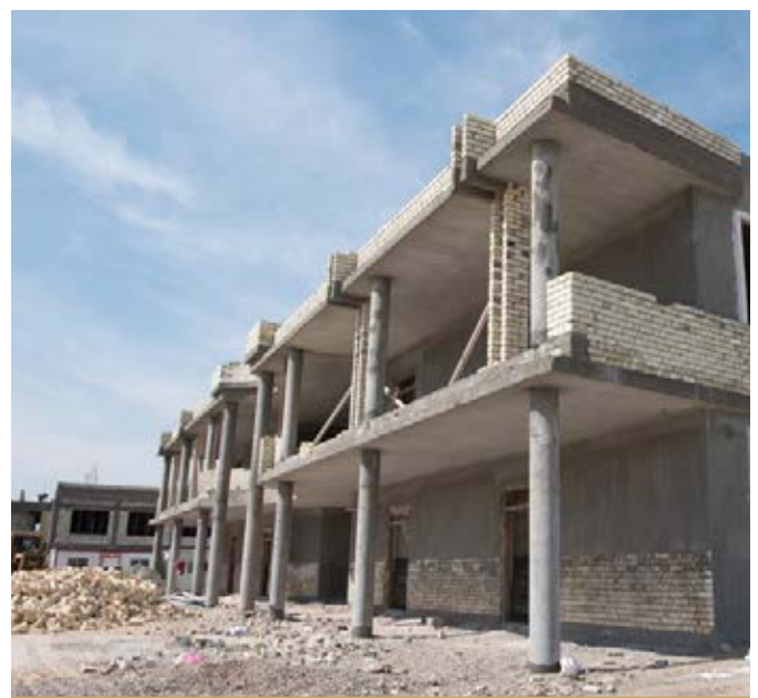
THE LABORATORY BUILDING FOR THE VETERINARY COLLEGE, WHICH IS BEING REHABILITATED BY FFS.
