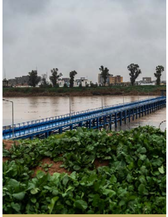
AFTER: THE REHABILITATED INTAKE AT THE DANEDAN WATER TREATMENT PLANT IN WEST MOSUL. NOW THAT THE PROJECT IS COMPLETE, THE PLANT SERVES SOME 55,000 RESIDENTS.
