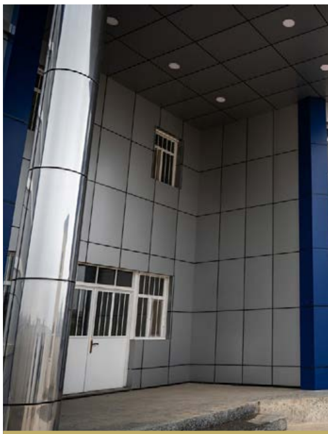
THE OUTSIDE OF THE AL KARAMA POLICE STATION. THE REHABILITATION OF THE POLICE STATION WAS COMPLETED IN 2018.
