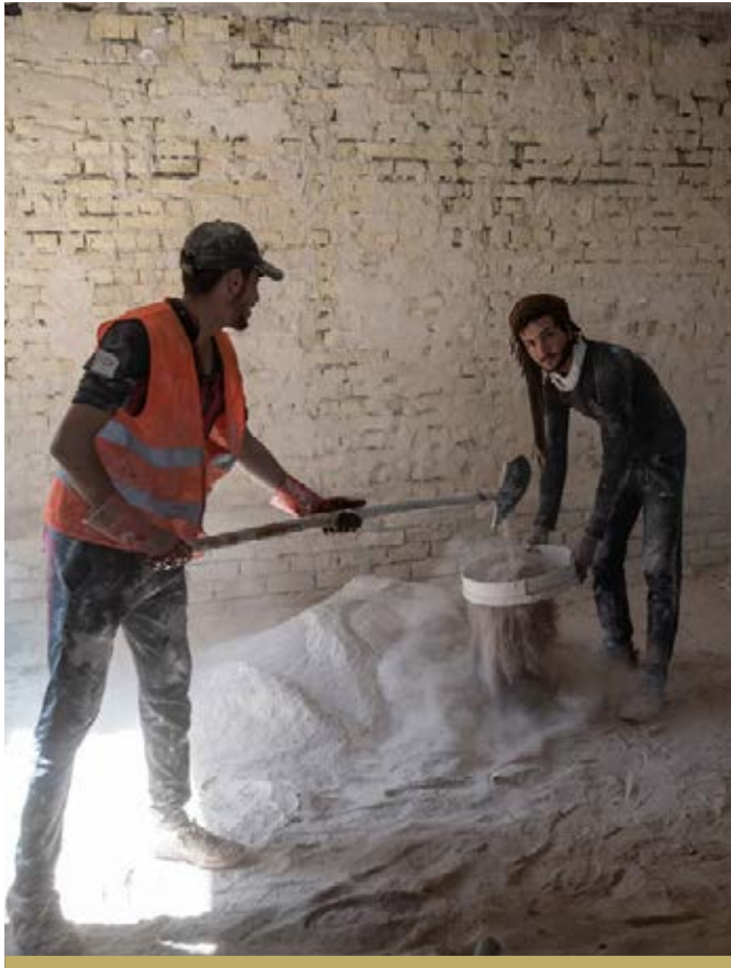
WORK IS ONGOING AT BAIJI'S CENTRAL PHC, WHICH WAS 83% COMPLETE AT THE END OF THE YEAR.
