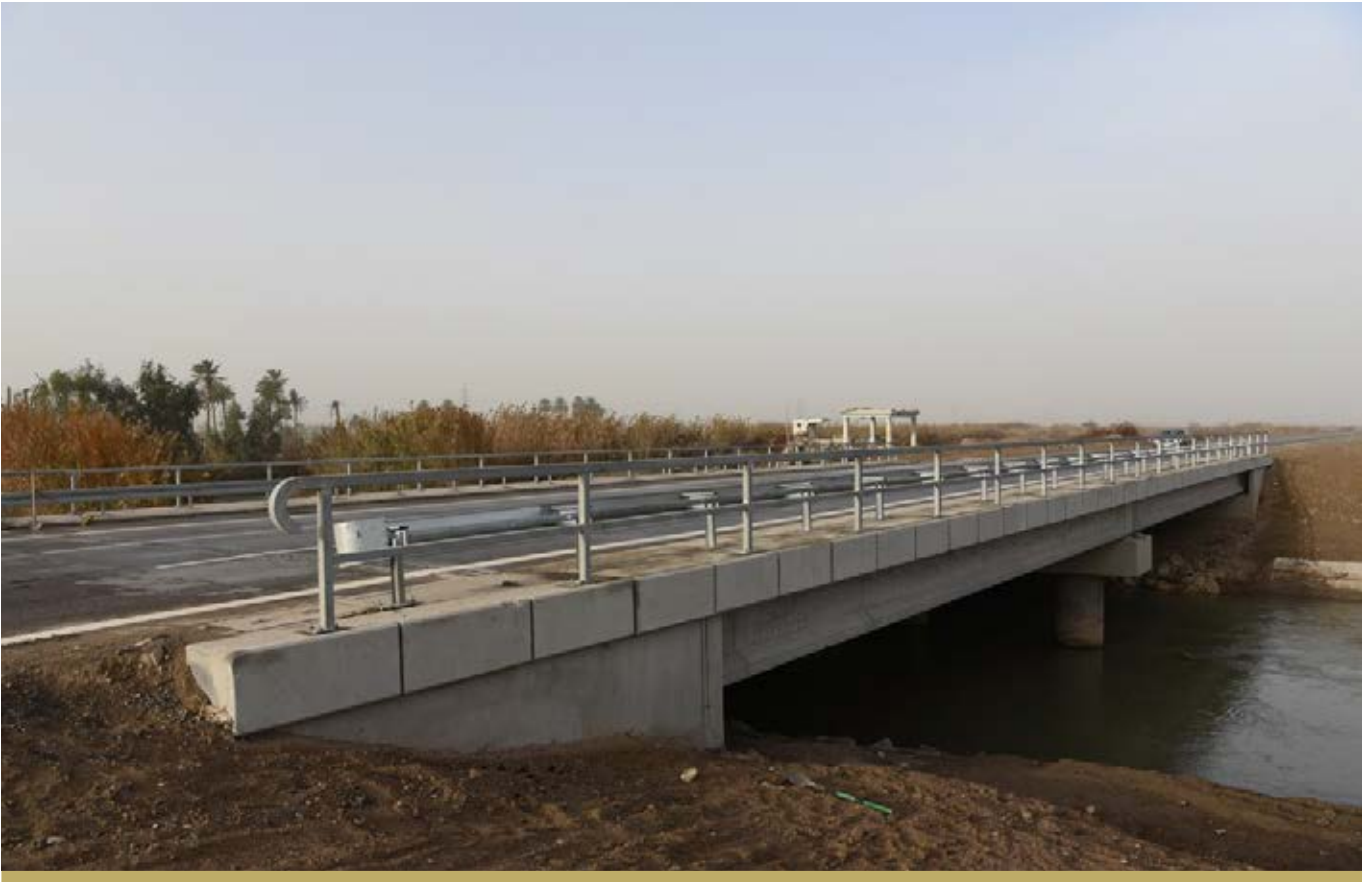
THE KARMA RIVER CONCRETE BRIDGE WAS ALMOST COMPLETE BY THE END OF 2018.
