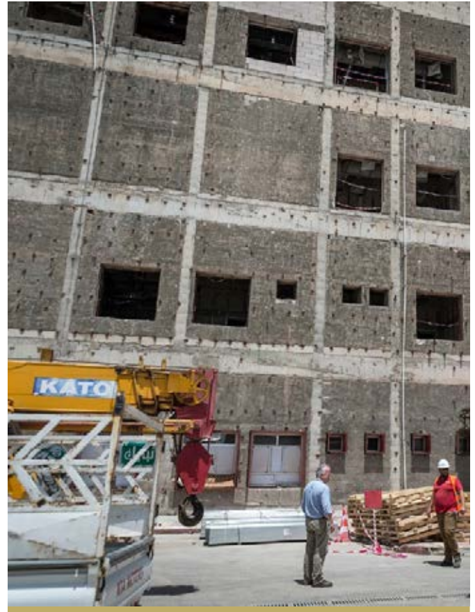
AFTER: WORK IS ONGOING TO REPAIR THE FAÇADE OF THE BUILDING, AS WELL AS THE INTERIOR.
