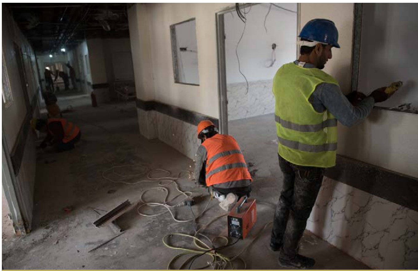
WORK IS ONGOING INSIDE THE RAMADI MATERNITY HOSPITAL, WHICH WAS 18% COMPLETE BY THE END OF THE YEAR.
