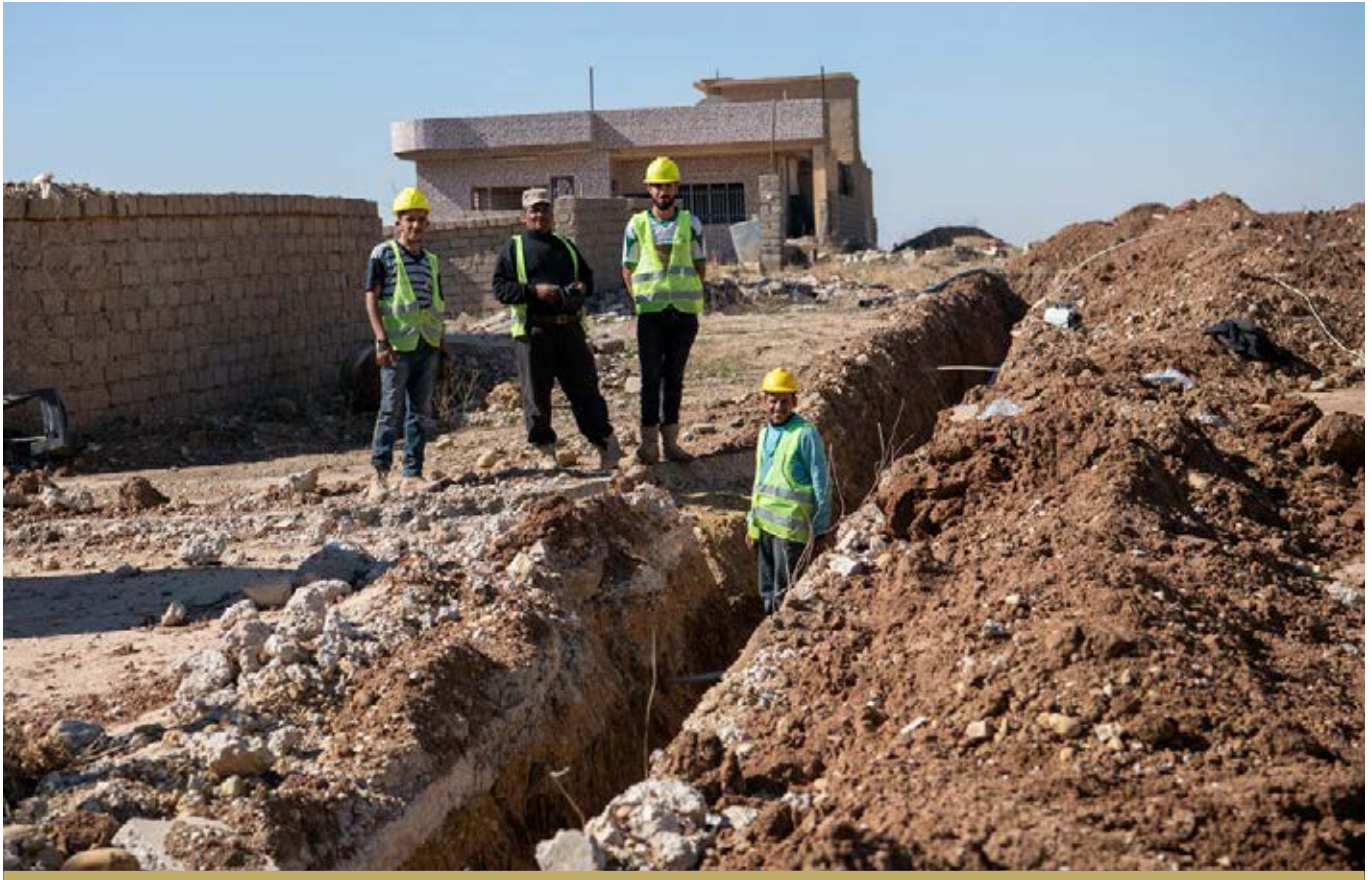
A PROJECT TO REHABILITATE THE WATER NETWORK IN BATNAYA WAS ONGOING IN 2018.
