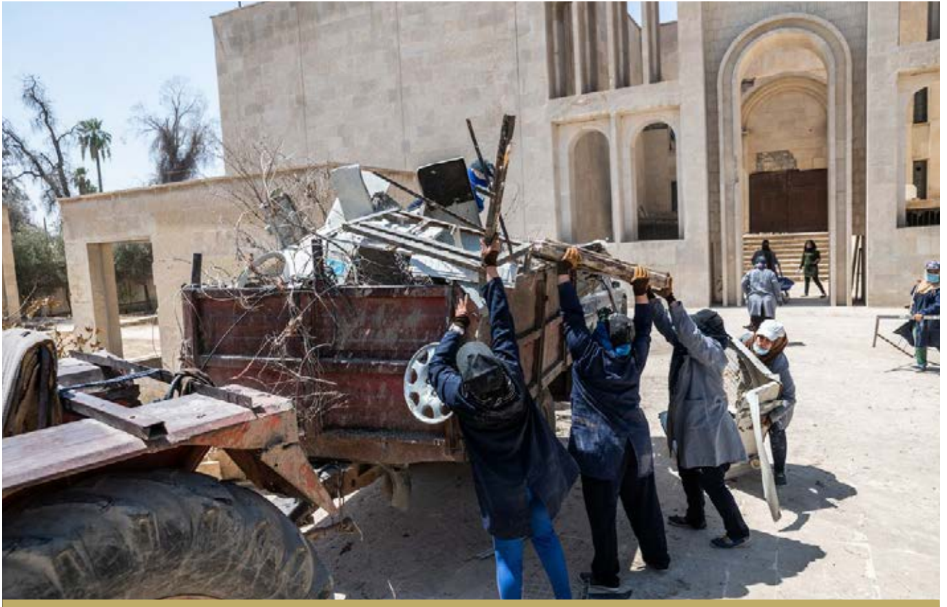
MEMBERS OF AN FFS CASH FOR WORK TEAM CLEAR RUBBLE AND DEBRIS FROM OUTSIDE THE MOSUL MUSEUM IN WEST MOSUL.
