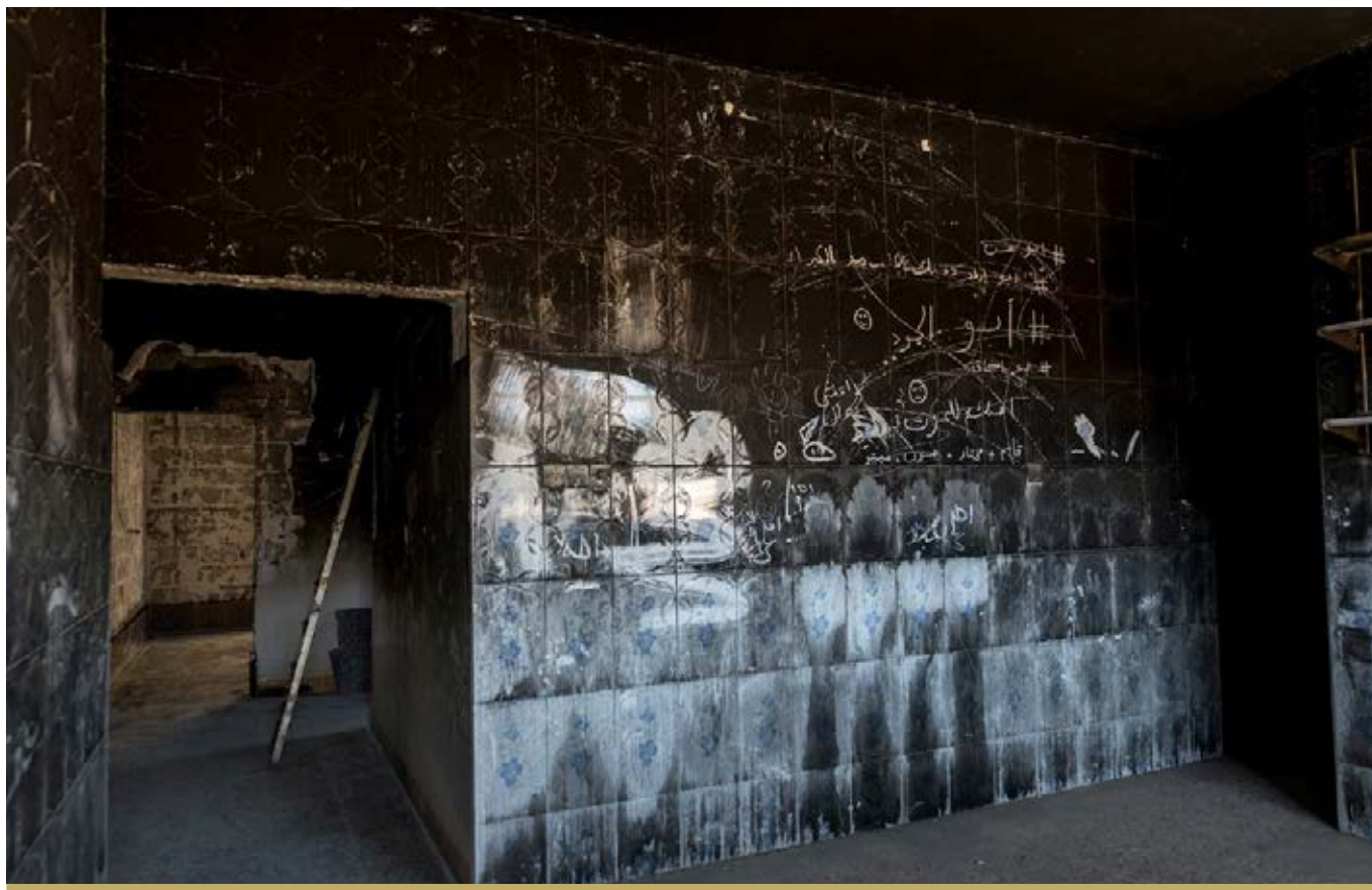
BEFORE: HOUSES IN BOTH BARTELA AND BASHIQA WERE SEVERELY DAMAGED. THIS EXAMPLE SHOWS EXTENSIVE BURNING INSIDE A HOME.
