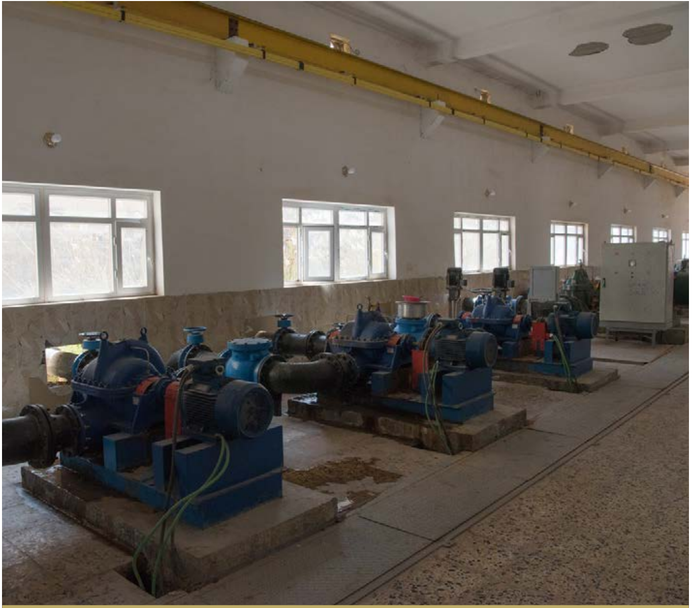
WATER PUMPS AT THE AL AZRAGIYAH WATER COMPLEX IN FALLUJAH, REHABILITATED IN 2017. PRIOR TO REHABILITATION IT WAS NOT FUNCTIONAL, BUT NOW IT SERVES 60% OF THE FALLUJAH POPULATION.
