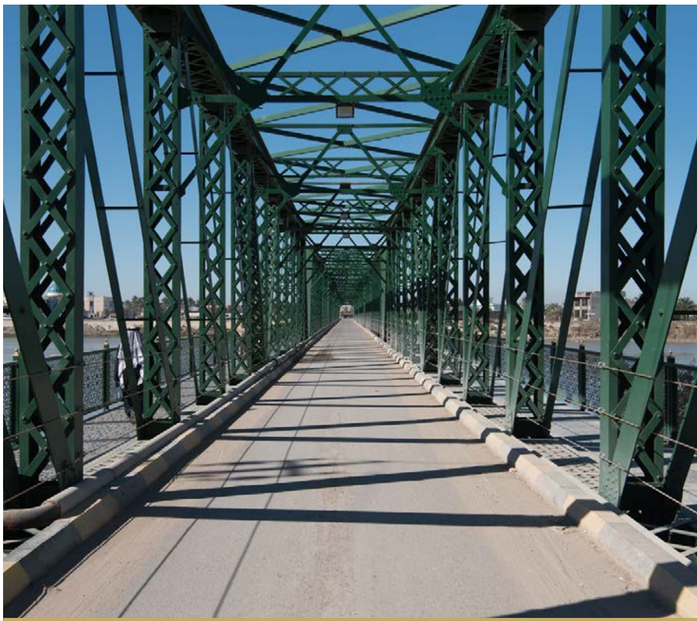
THE ICONIC FALLUJAH IRON BRIDGE. THE REHABILITATION OF THE BRIDGE BY FFS WAS COMPLETED IN 2018.
