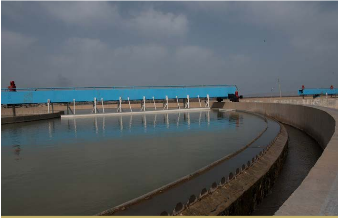
SEDIMENTATION TANKS AT BAIJI'S CENTRAL WATER TREATMENT PLANT. THE TANKS WERE REHABILITATED IN 2018 AS PART OF PHASE ONE OF THE REHABILITATION OF THE FACILITY.
