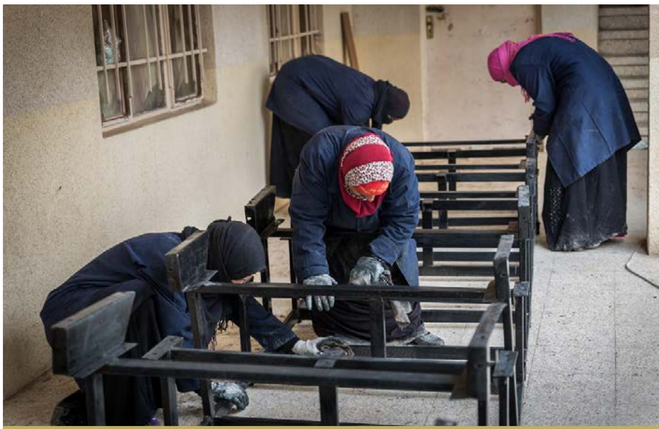
WOMEN WORK REPAIRING DESKS AS PART OF THE CASH FOR WORK PROJECT. SIXTEEN WOMEN WORKED TO REPAIR 500 DESKS.
