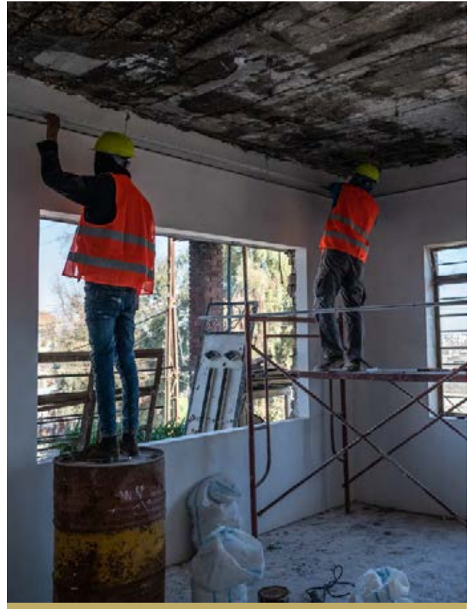
WORK IS UNDERWAY TO REHABILITATE A FAMILY HOME IN THE WADI HAJAR NEIGHBOURHOOD OF WEST MOSUL.
