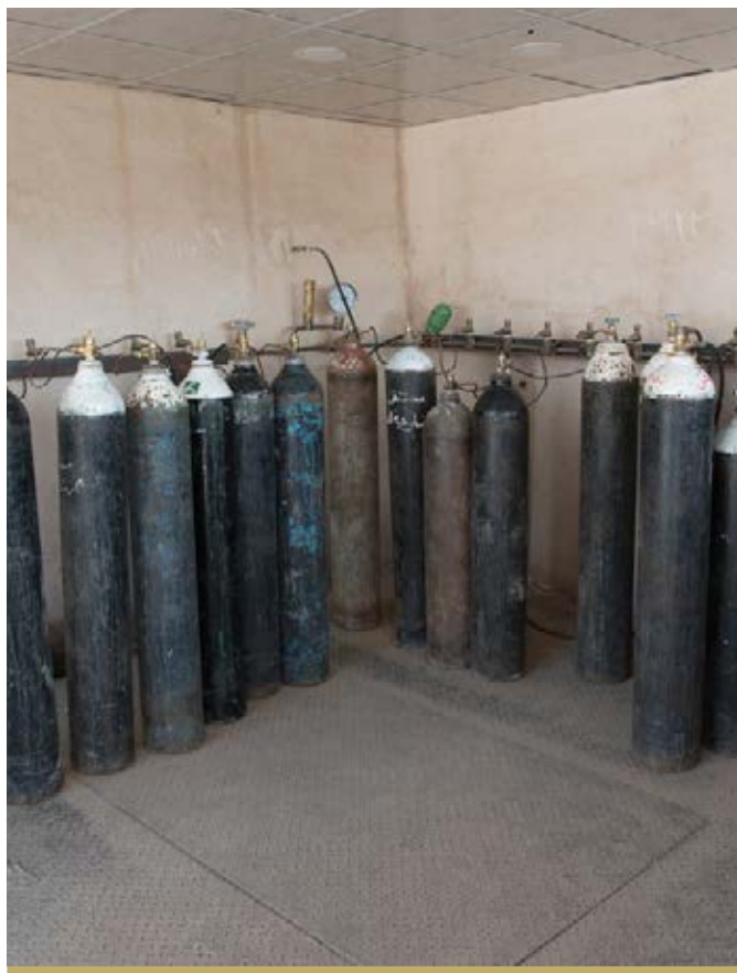
OXYGEN GAS CANISTERS AT THE MEDICAL OXYGEN GAS PLANT.
