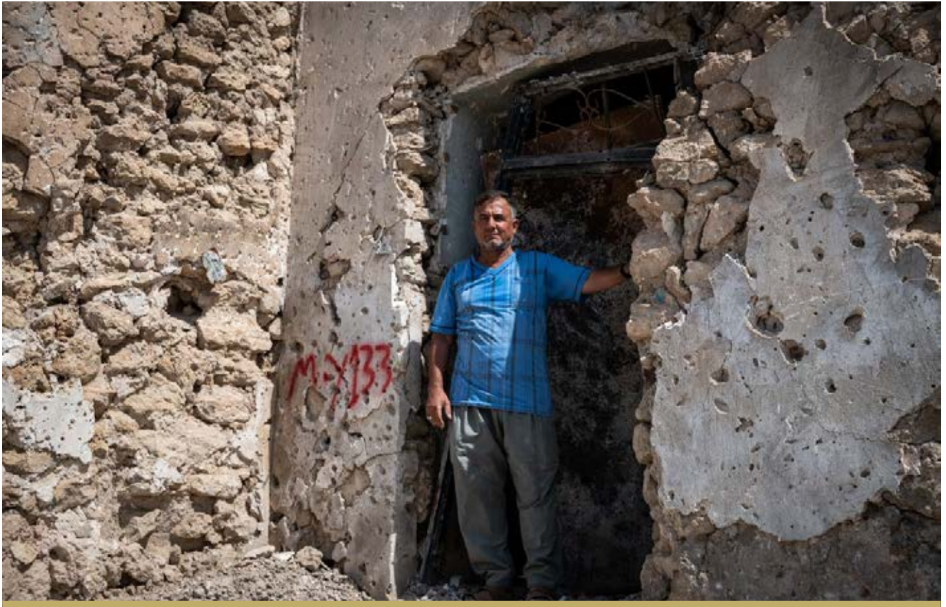
YOUSSEF SHWBAIL IS PICTURED OUTSIDE HIS DAMAGED HOME IN MOSUL'S OLD CITY. MR. SHWBAIL'S HOME WILL BE REHABILITATED BY FFS IN 2019.
