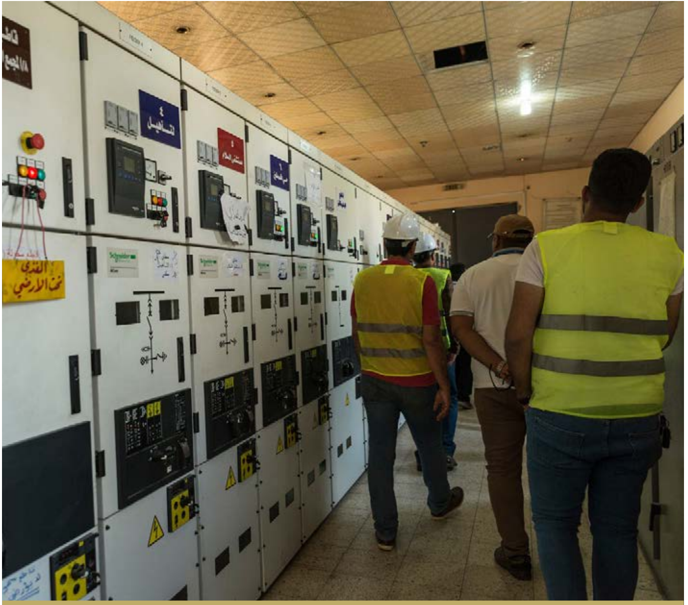
NOW THAT THE MUJAMMAH SIHY SUBSTATION IN EAST MOSUL IS COMPLETE, IT IS PROVIDING ELECTRICITY FOR 35,000 PEOPLE.
