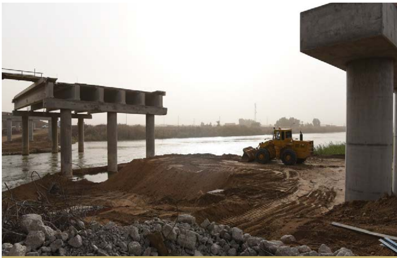
WORK IS UNDERWAY ON THE PALESTINE CONCRETE BRIDGE IN RAMADI, FFS'S LARGEST BRIDGE PROJECT IN ANBAR.
