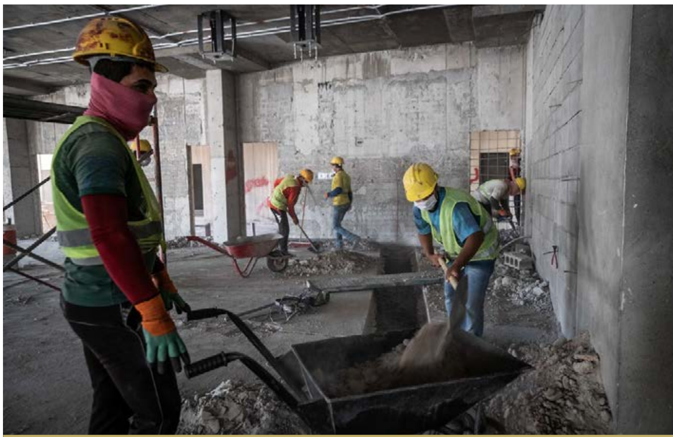
WORK IS UNDERWAY AT TIKRIT TEACHING HOSPITAL, THE LARGEST FFS PROJECT IN IRAQ.
