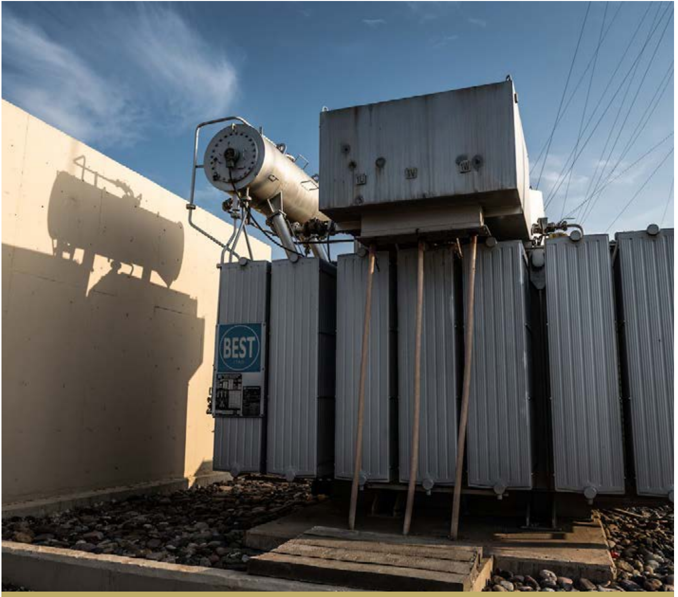
THE ALARBAJEYA SUBSTATION IN EAST MOSUL, WHICH WAS COMPLETED IN 2018.
