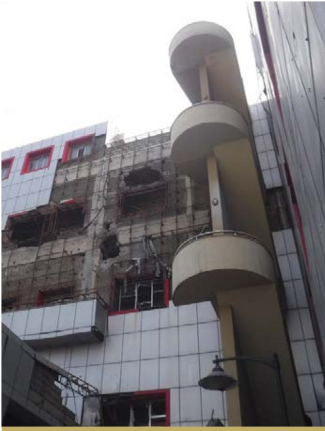
BEFORE: THE FAÇADE OF QAYARA HOSPITAL PRIOR TO THE BEGINNING OF REHABILITATION WORKS.
