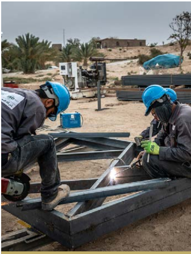
WORK IS UNDERWAY TO REHABILITATE AL KHOOR BRIDGE NEAR THE TOWN OF AL QAIM. THE PROJECT WAS 64% COMPLETE BY THE END OF THE YEAR.
