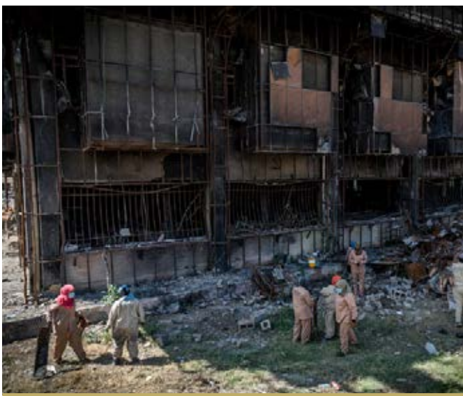
A CFW TEAM CLEARS RUBBLE AND DEBRIS FROM AROUND THE CENTRAL LIBRARY AT THE UNIVERSITY OF MOSUL.
