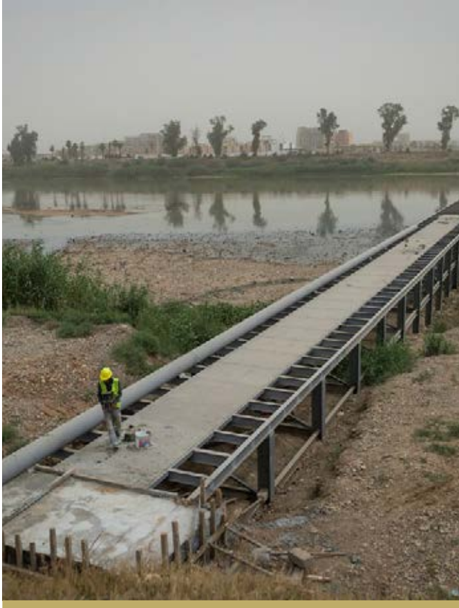
BEFORE: THE INTAKE AT THE DANEDAN WATER TREATMENT PLANT IN WEST MOSUL.
