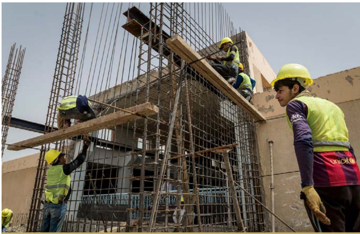
WORK IS ONGOING IN WEST MOSUL ON THE NEW WATER TREATMENT PLANT. THE NEW WTP IS THE LARGEST IN THE CITY AND, WHEN COMPLETED, IT WILL PROVIDE WATER FOR CLOSE TO ONE MILLION PEOPLE.
