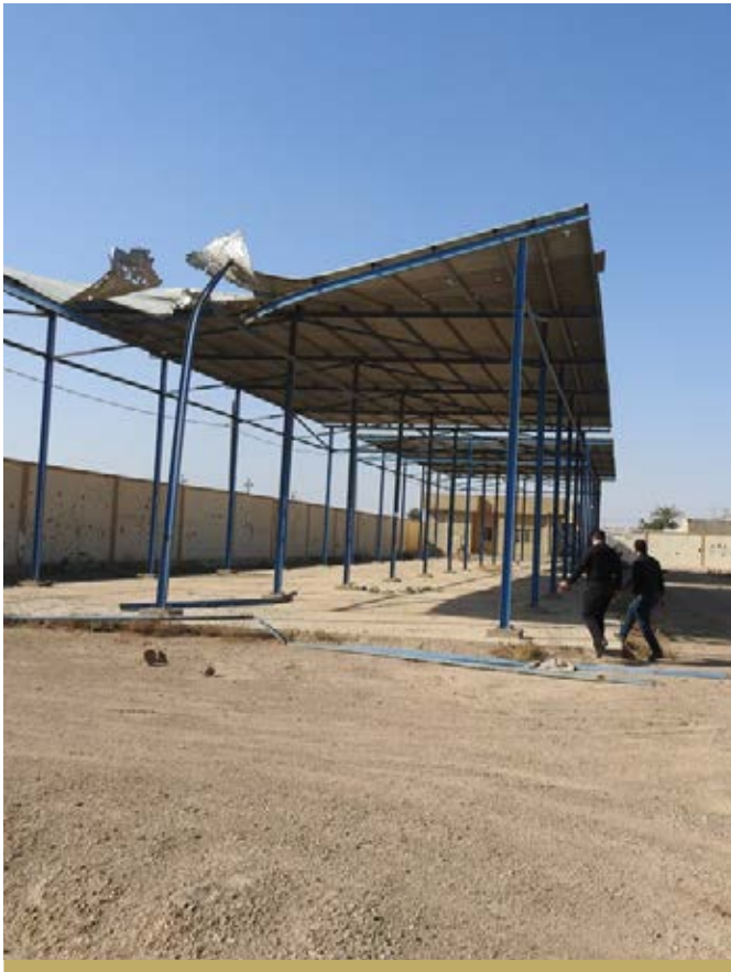
BEFORE: THE MUNICIPAL WORKSHOPS IN FALLUJAH PRIOR TO REHABILITATION.
