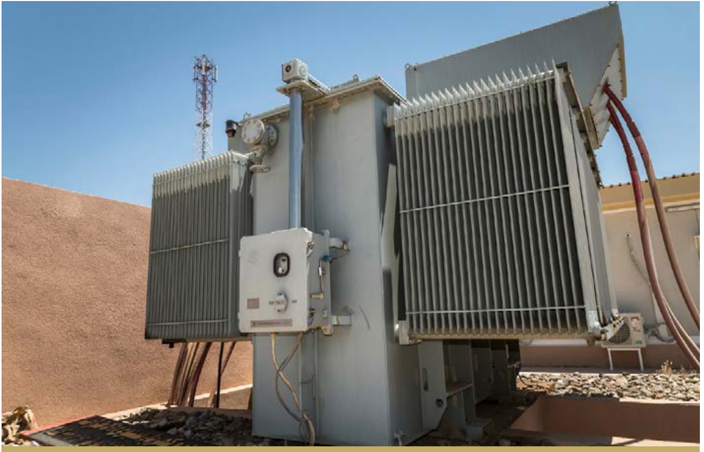
PART OF THE SUBSTATION IN TELESKOF, REHABILITATED IN 2018 BY FFS.
