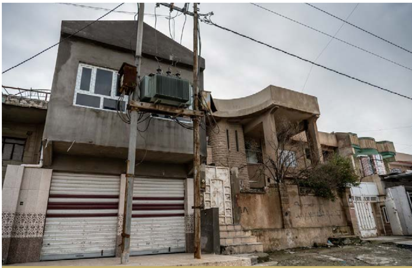
A DISTRIBUTION TRANSFORMER IN WEST MOSUL. 200 OUTDOOR DISTRIBUTION TRANSFORMERS WERE SUPPLIED IN WEST MOSUL IN 2018.
