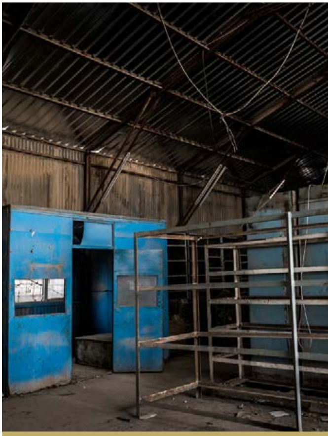
BEFORE: A WAREHOUSE AT THE OIL AND FUEL DEPOT IN WEST MOSUL, PRIOR TO ITS REHABILITATION.
