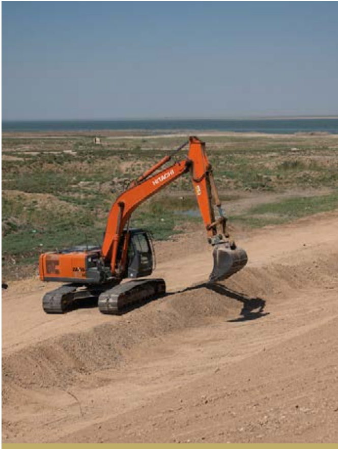
WORK IS ONGOING AT THE HAMRIN DAM AND THE PROJECT WAS 12% COMPLETE BY THE END OF THE YEAR.
