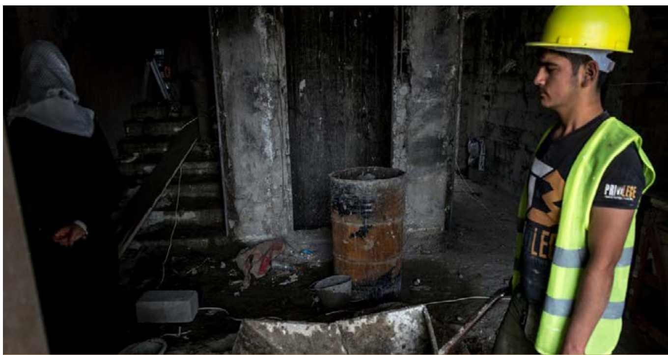
THE ELECTRICITY DISTRIBUTION DIRECTORATE BUILDING IN EAST MOSUL WAS HEAVILY DAMAGED DURING THE BATTLE TO LIBERATE THE CITY.
