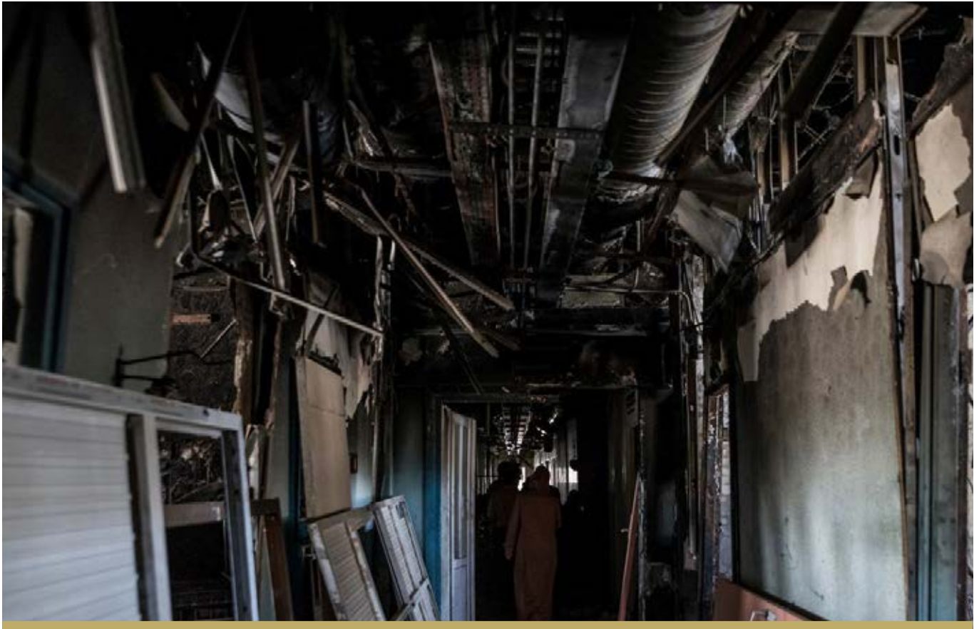
DURING THE 2018 YEAR, THE ASSESSMENT AND DESIGN FOR AL KHANSA MATERNITY HOSPITAL WAS COMPLETED BY THE FFS, ALTHOUGH THE PROJECT REMAINS UNFUNDED.
