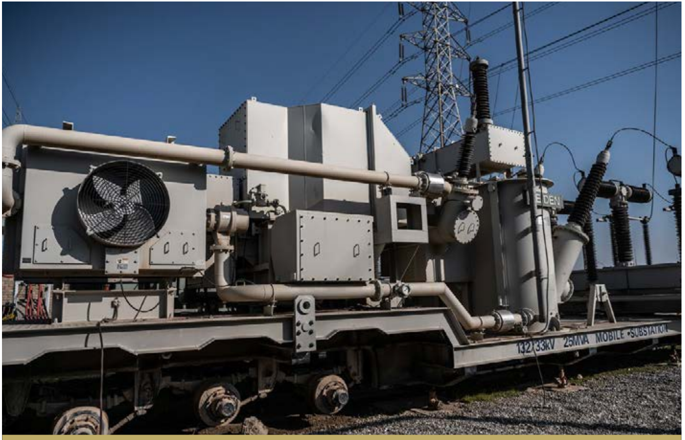
WEST MOSUL 132KV MOBILE SUBSTATION, WHICH WAS 63% COMPLETE BY THE END OF 2018.
