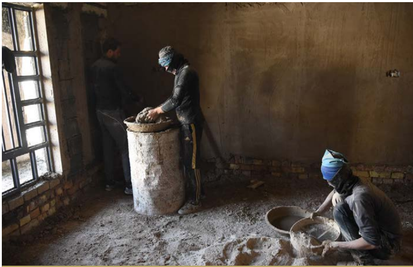
WORKERS ON SITE AT A HOUSING PROJECT IN RAMADI. IN TOTAL, FFS HAS UNDERTAKEN 22 HOUSING PROJECTS IN THE CITY. BY THE END OF 2018 ALL BUT ONE WERE COMPLETED.
