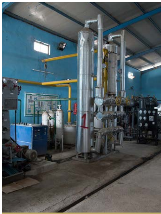
THE INSIDE OF THE MEDICAL OXYGEN GAS PLANT AT THE TIKRIT TEACHING HOSPITAL, WHICH WAS REHABILITATED IN 2018
