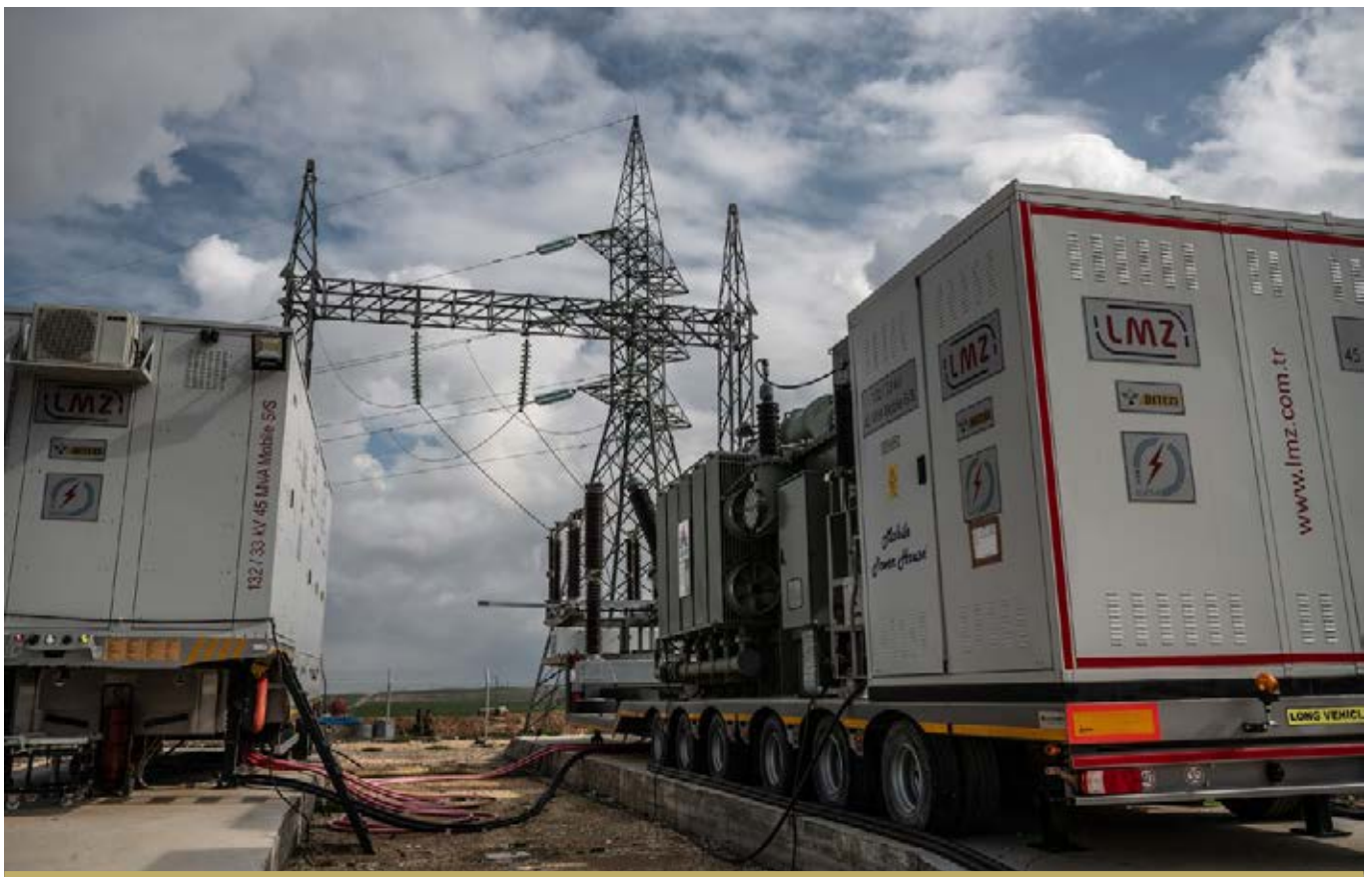
THE 132/33 KV MOBILE SUBSTATION INSTALLED IN SINUNI DURING 2018.
