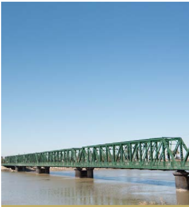
THE FALLUJAH IRON BRIDGE. THE REHABILITATION OF THE BRIDGE WAS COMPLETED IN 2018.
