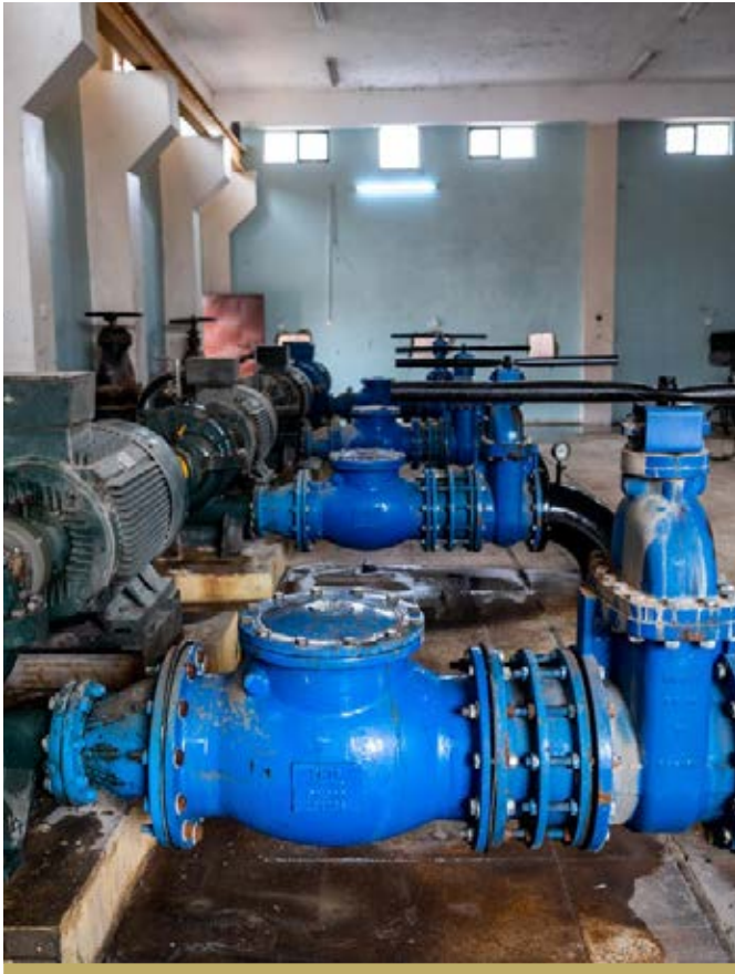
WORK HAS BEEN COMPLETED AT THE AL SAHIRON WATER TREATMENT PLANT IN EAST MOSUL.
