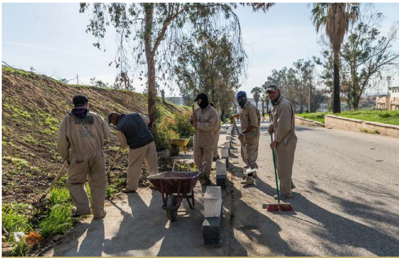
MEMBERS OF A CASH FOR WORK TEAM CLEAR A ROAD AT THE ENTRANCE TO THE NORTHERN TECHNICAL UNIVERSITY IN EAST MOSUL.
