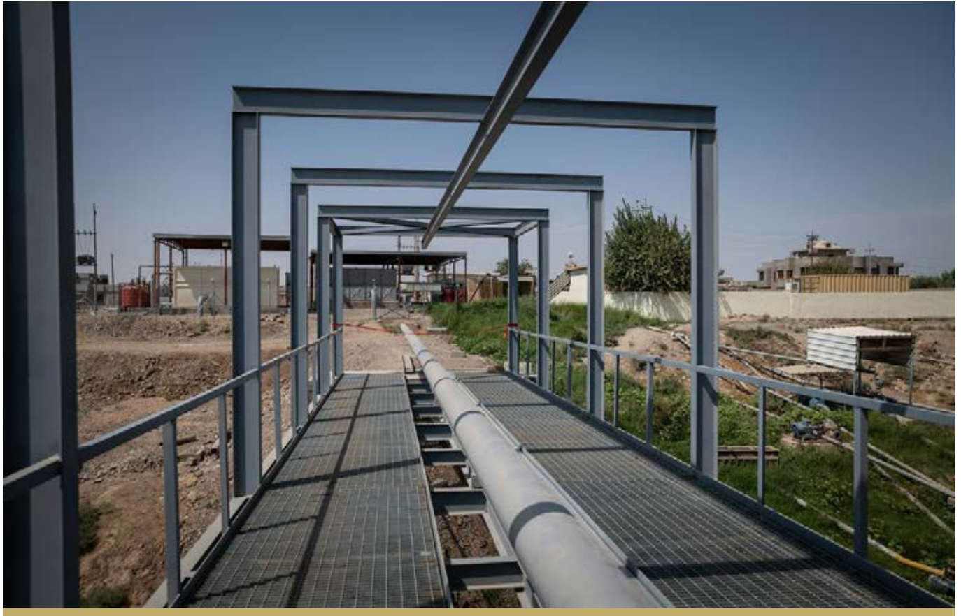
WORK AT THE AL HOD WATER TREATMENT PLANT STOOD AT 70% COMPLETION AT THE END OF THE YEAR.
