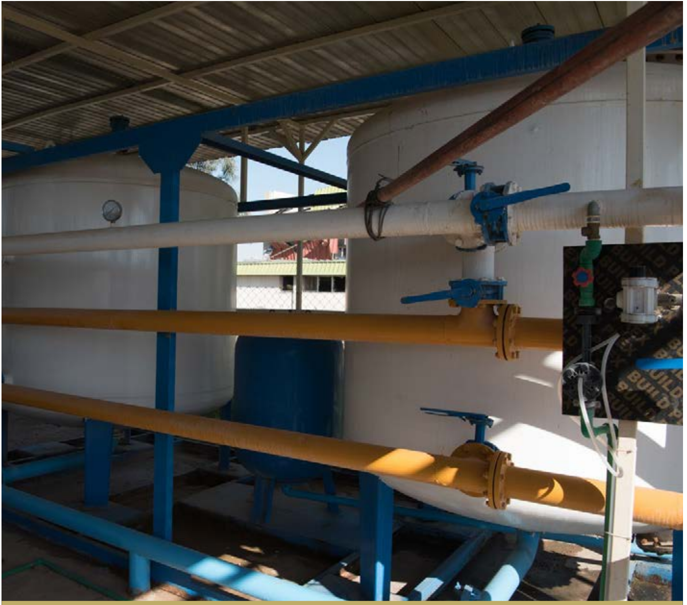
THE WATER TREATMENT PLANT AT THE ANBAR TECHNICAL INSTITUTE, REHABILITATED IN 2018. PRIOR TO ITS REHABILITATION, THERE WAS NO SOURCE OF WATER ON CAMPUS.
