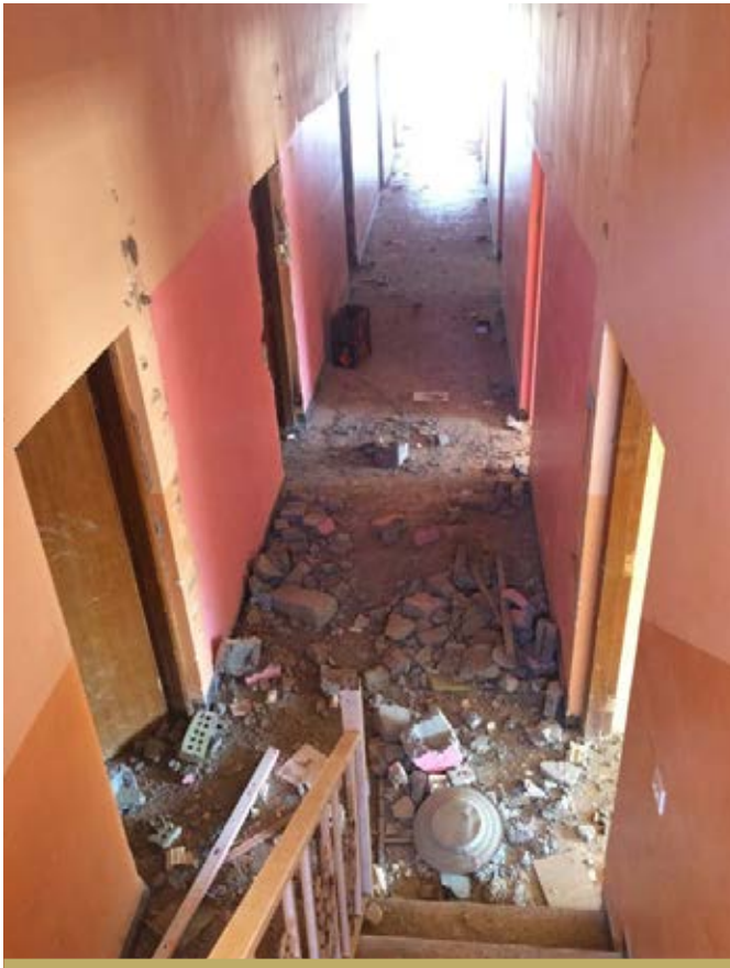
BEFORE: THE HALLWAY OF THE GIRLS' HOSTEL AT WOMEN'S DORMITORY, ANBAR TECHNICAL INSTITUTE.
