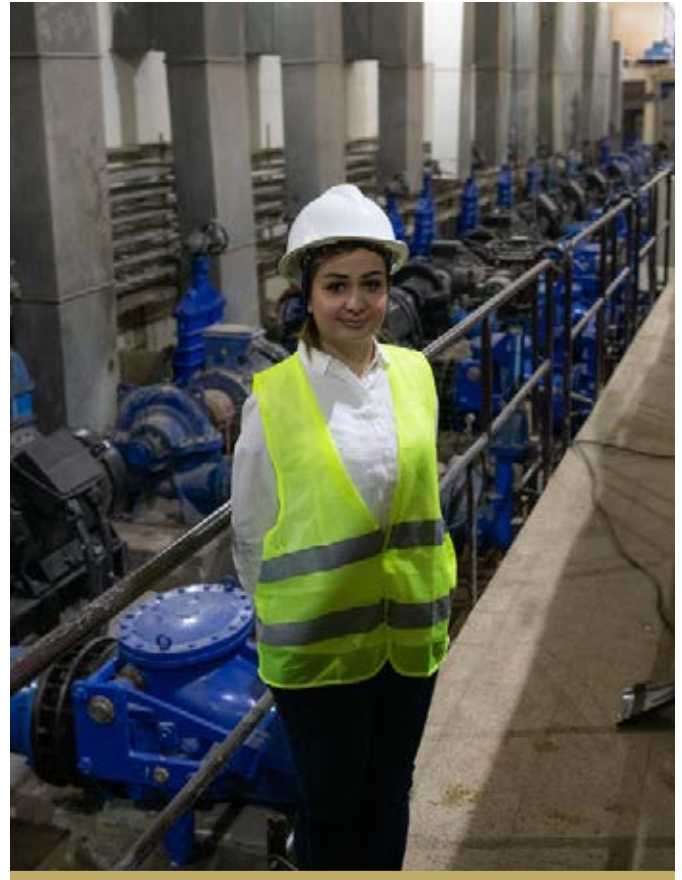
FFS ENGINEER SAHAR STANDS FOR A PHOTO IN THE PUMP ROOM AT AL QUBBA WATER TREATMENT PLANT IN EAST MOSUL. WORK AT AL QUBBA WAS 73% COMPLETE AT THE END OF 2018.
