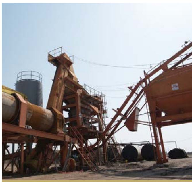
PART OF THE HEET ASPHALT FACTORY, JUST OUTSIDE THE CITY, WHICH WAS REHABILITATED BY THE FFS IN 2018.
