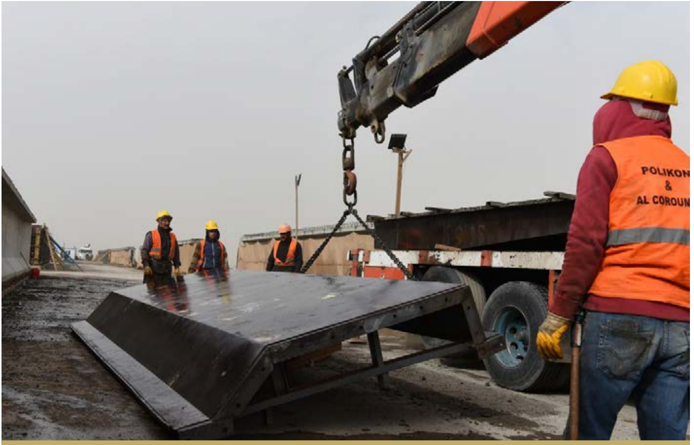
WORK AT THE PALESTINE CONCRETE BRIDGE IN RAMADI IS ONGOING. THE BRIDGE IS THE BIGGEST ROADS AND BRIDGES SECTOR PROJECT IN ANBAR.
