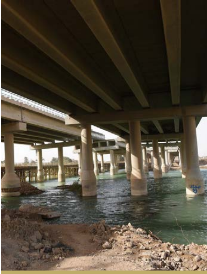
THE PALESTINE CONCRETE BRIDGE IN RAMADI, WHICH IS LARGEST BRIDGE PROJECT IN ANBAR.
