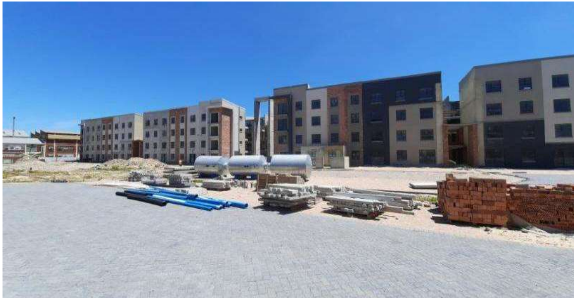
Figure 1: E-Junction Residential Development during the construction phase. Three solar storage tanks in the foreground before installation.
